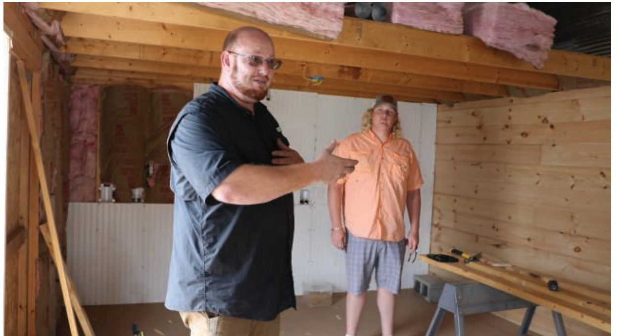
ELIZABETH WONG BARNSTEAD | WKC Micah Seavers (foreground), and Buck Shelton, both co-directors of Camp G.R.A.V.E.S. in Graves County, Ky., stand inside a tiny home under construction on July 19, 2022.
