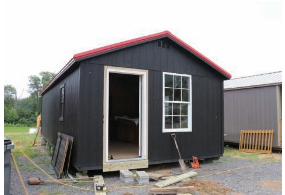
ELIZABETH WONG BARNSTEAD | WKC A tiny home in progress is seen at Camp G.R.A.V.E.S. in Graves County, Ky., on July 19, 2022.
